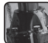
Seal Damage & Leaks
